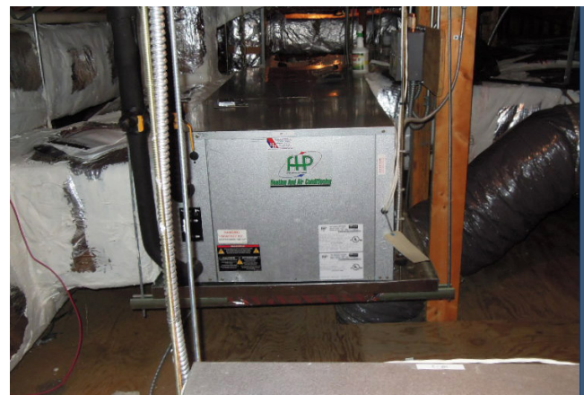
Four 6 ton Bosch FHP horizontal geothermal heat pumps serve the 9,000 sq ft Kentlands Community Center to provide abundant heating and cooling
