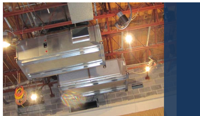
Bosch FHP LV Series 8 and 10 ton commercial heat pumps installed in the ceiling of the auditorium. connect into existing ductwork system to provide year-round comfort
