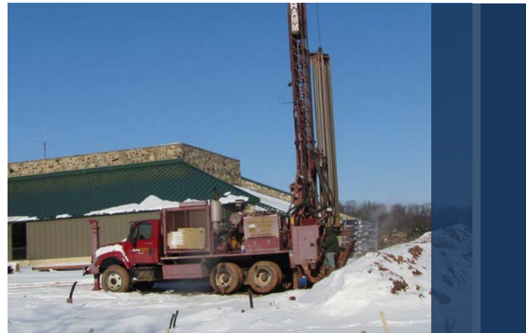
Twenty wells each 300 ft deep provide a closed-loop geothermal field routed to the mechanical room.
